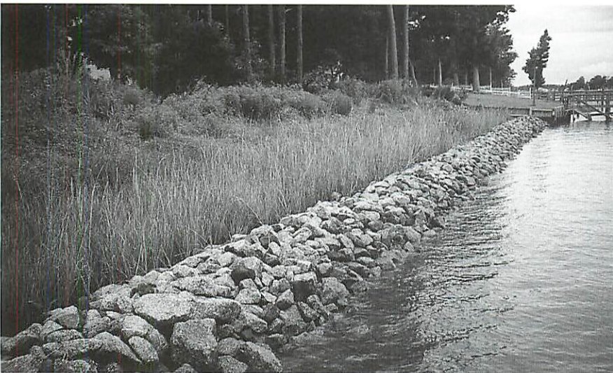
Figure 16, top: Rock sills and graded shoreline, ready for vegetative planting. Figure 17, bottom: Completed rock sills with healthy marsh grass sheltered from waves.
