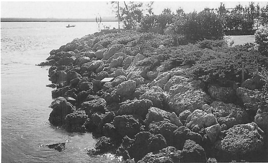
Figure 20, top: Preparation for a sloping rock revetment in construction phase. Figure 21, bottom: Marine limestone used in sloping rock revetment.
