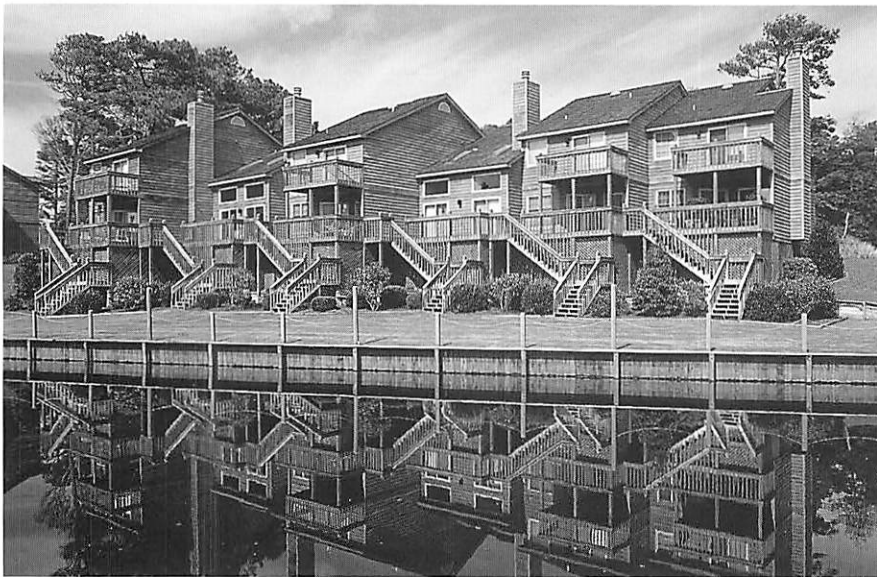
Figure 18, top: Vertical wooden bulkhead retaining weight of soil landward. Note lack of any fringing marshes and scour areas. Figure 19, bottom: Vertical wooden bulkhead in front of housing units.
