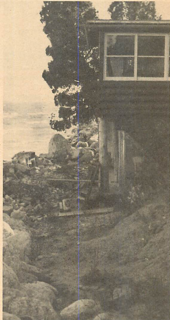
Erosion and high lake levels on Lake Michigan have taken their toll on this summer home in Oostburg, Wisconsin.
