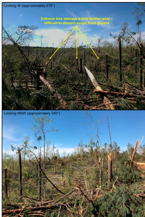
FIG. 3. Images of severe tree damage found by the UAH ground survey team along Brown Taylor Road NNE of the GWX radar. (top) What appeared as likely extreme tree damage just west of the road is noted.
