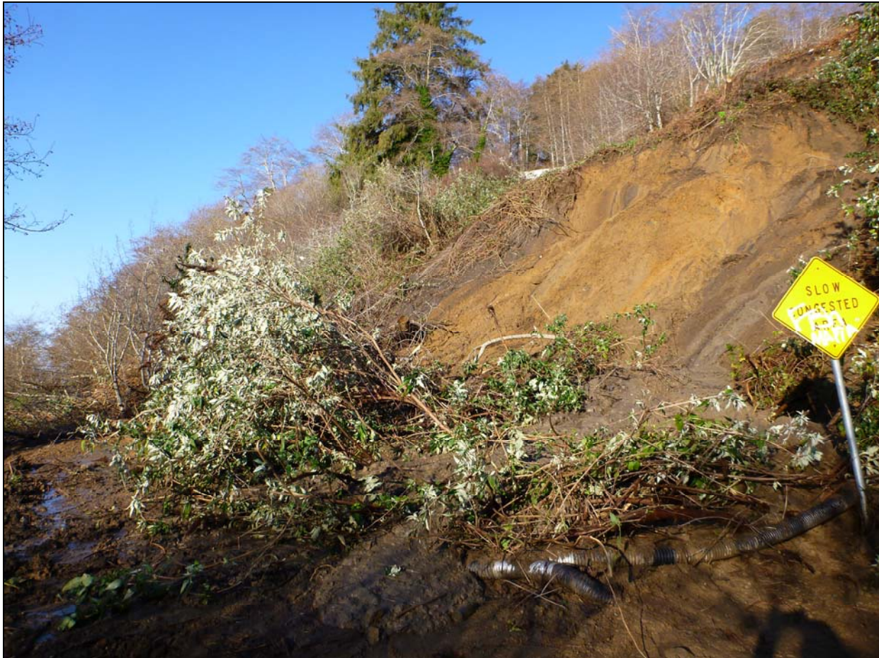
Figure 6. Recent debris slide (January 2012) blocking the Requa Road which provides access to the Requa Resort.
