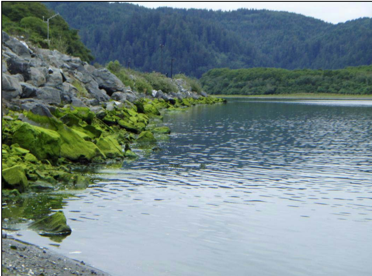
Figure 12. Looking upstream at riprap installed with FEMA grant funds to protect the campground and boat launch area. The satellite antenna (grey pole on left) for the Yurok Tribe's lower estuary gaging station provides a marker for the location map.
