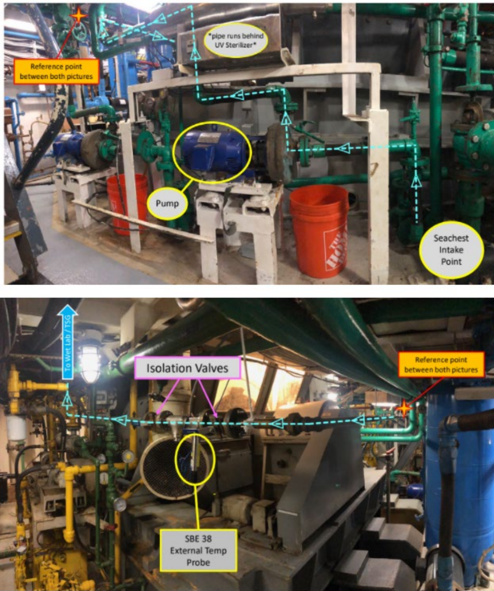
Figure 4. Flow diagram of Scientific Seawater System through the bow thruster room from the seachest intake point (top) to the output into the wet lab/TSG (bottom). Photo: SST Wilkins.
