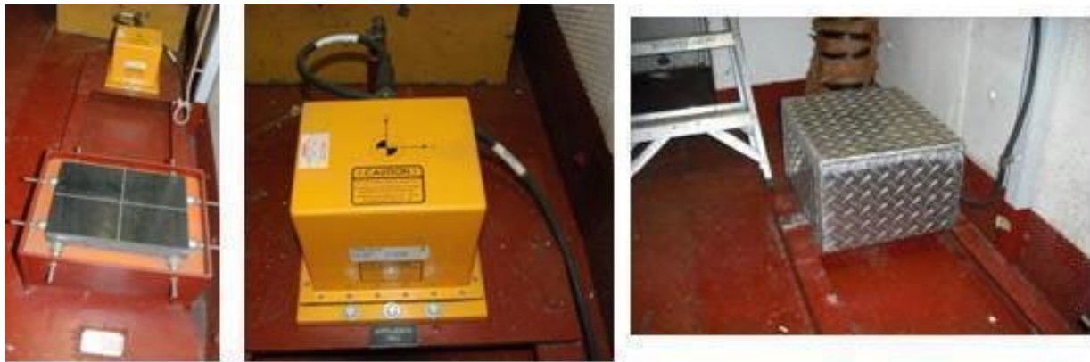
Figure 2. IMU and granite block (left), IMU (center), IMU under protective housing (right). All photos in the fan room.
