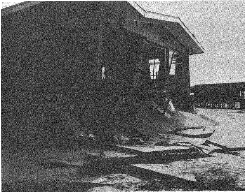
Figure III-21 Example of Slab on Grade Failure as a result of underming by wave action. Note the building to the right surviving intact on Pile Foundation. Hurricane Eloise (49).
