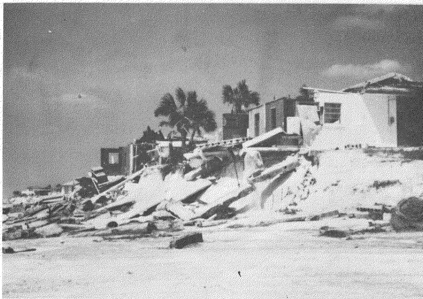
Figure III-20. Structural Failures Caused by Undermining Wave Action. Panama City Beach, Hurricane Eloise (9/75)
