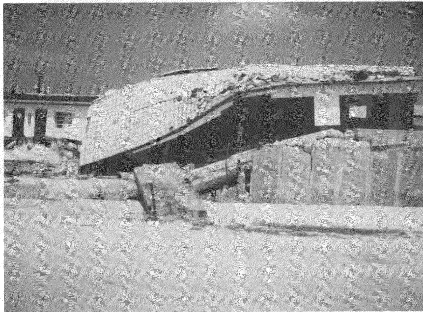
Figure IV-12. This seawall failed to prevent sand erosion from behind the wall and subsequent failure of the slab and supported building, Hurricane Eloise, (9/75).
