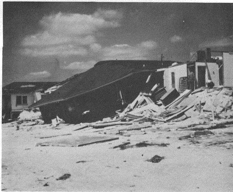
Figure IV-10. Slab Failures Due to Undermining of Concrete Floor Slabs Poured on Grade. Hurricane Eloise 9/75.
