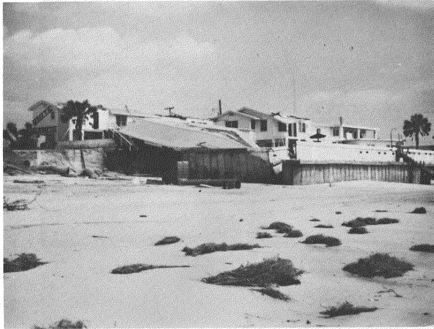
Figure IV-11. Seawall Construction did not prevent sand from washing out from behind it resulting in structural failure of the building, Hurricane Eloise (9/75).
