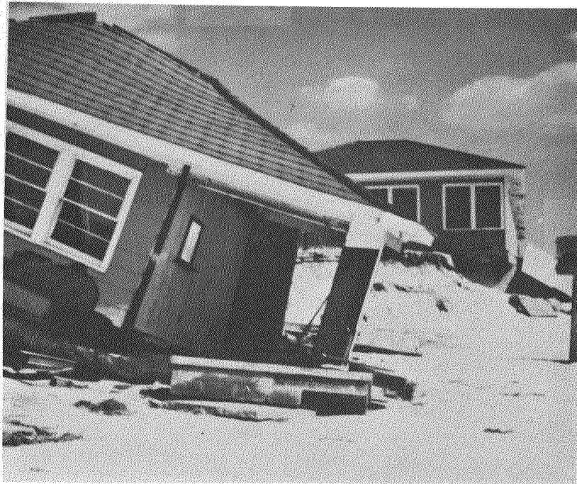
Figure IV-9. Slab Failure Due to Undermining Action. Hurricane Eloise 9/75.
