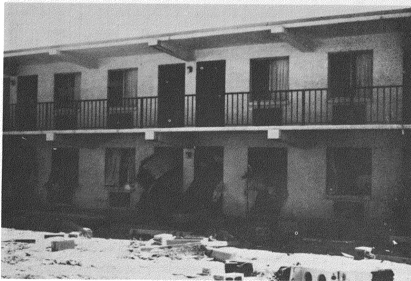
Figure III-8. Landward Side of a Motel Showing Furniture, Appliances and Other Non-Structural Debris Moved Through the Windows by Wave Forces. Hurricane Eloise (9/75)
