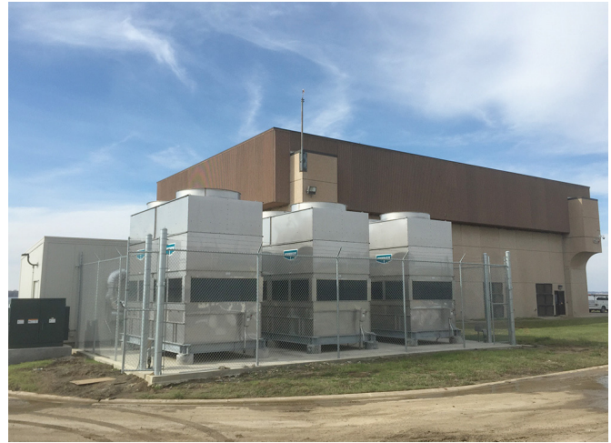
Drinking water cooling system. Source: WUCA.
