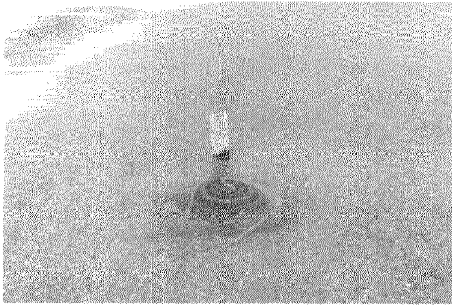
Figure 13. Clogged Roof Drain and Standing Water
