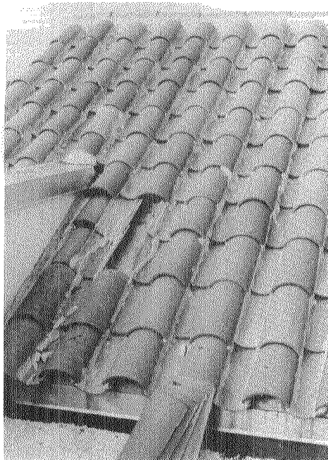
Figure 10. Roof Tiles Were Not Fastened Properly and Were Removed By Hand
