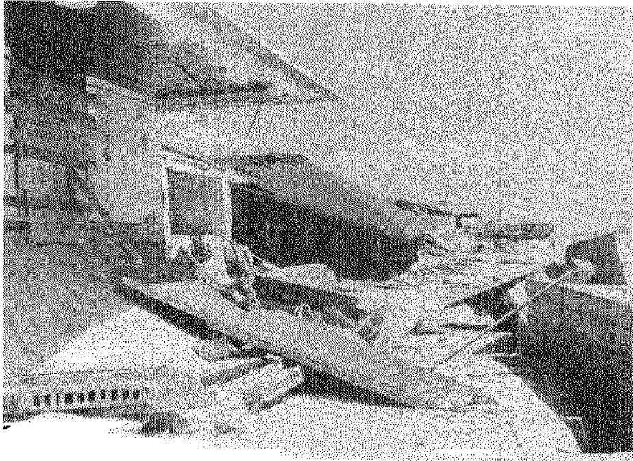
Figure 14. Structures with Spread Footings or Other Shallow Foundations Cannot Withstand Scour
