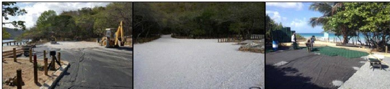
Figure 36. Examples of low impact development practices and permeable parking areas that allow for filtration of rain/run off (Photo source: Protectores de Cuencas)
