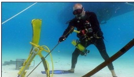
Figure 42. A diver installs a mooring buoy anchor system on the seafloor (Photo source: NOAA)
