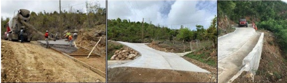
Figure 34. Example of road stabilization, including retaining wall (right) in USVI (Photo source: Coral Bay Community Council)
