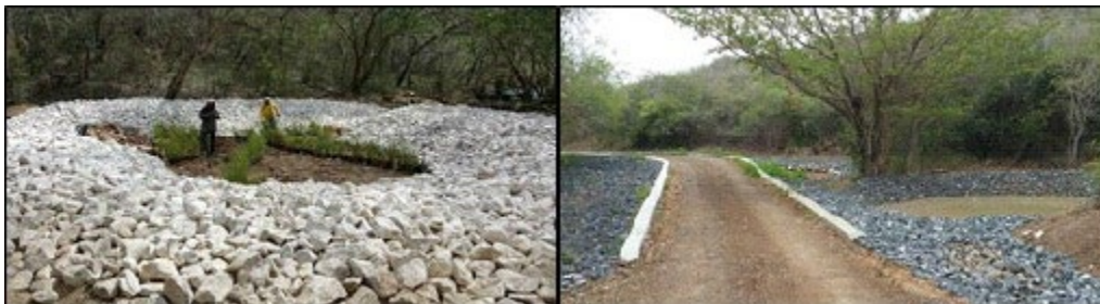
Figure 38. An example of sediment pond construction in Puerto Rico (Photo source: Protectores de Cuencas)
