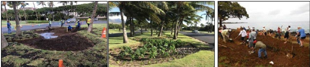
Figure 37. Bioretention area installation (left) and a rain garden (right) constructed in West Maui (Photo source: West Maui Ridge to Reefs)
