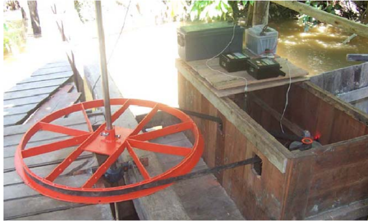
Figure 12: Single Stage Belted Gearing System, used on a Gorlov helical turbine in the Amazon River [29]
