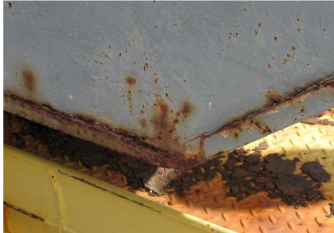
Figure 17: Used Pontoons Showing Rust Damage
