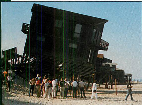
Inspecting Property Damage
