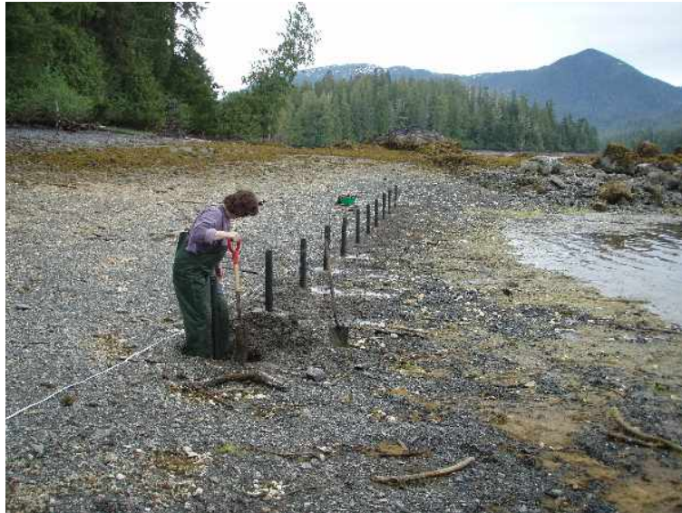
Figure 6. Construction of a fence for a flip-flop bag system. Note the fence wire used to orient placement of posts.
