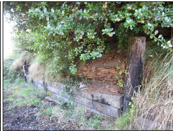
Figure 4. Deteriorating timber pile wall along the lower part of the beach access roadway. Note creosote pile.
