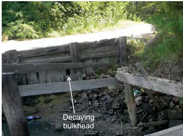
The bulkhead that supports the paved ramp leading to the dock is decaying and needs replaced.
