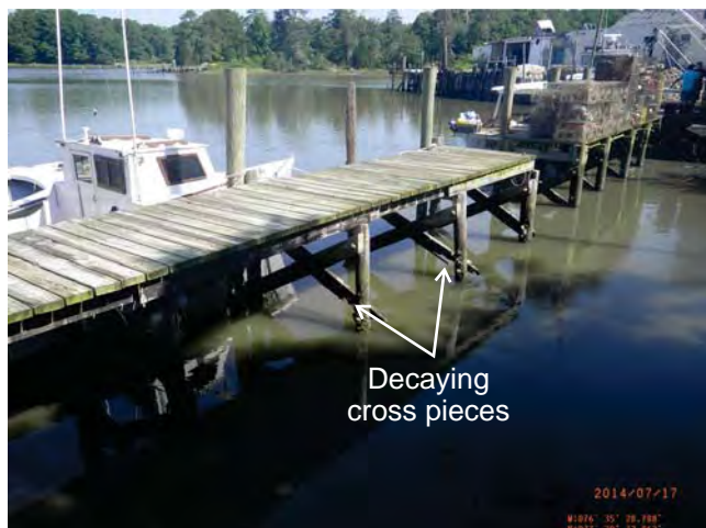
The L section of the docks have X braces that are in various stages of decay.
