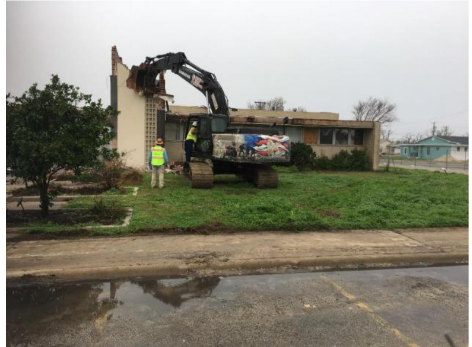
Photo: Demolition of the Aransas County Courthouse due to significant damage Source: William Whitson, LTRT
