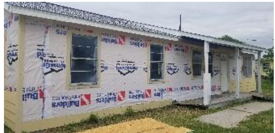
Top Photo: One of many houses destroyed during the hurricane Bottom Photo: Example of a house restored by volunteers Source: Aransas County Long Term Recovery Team
