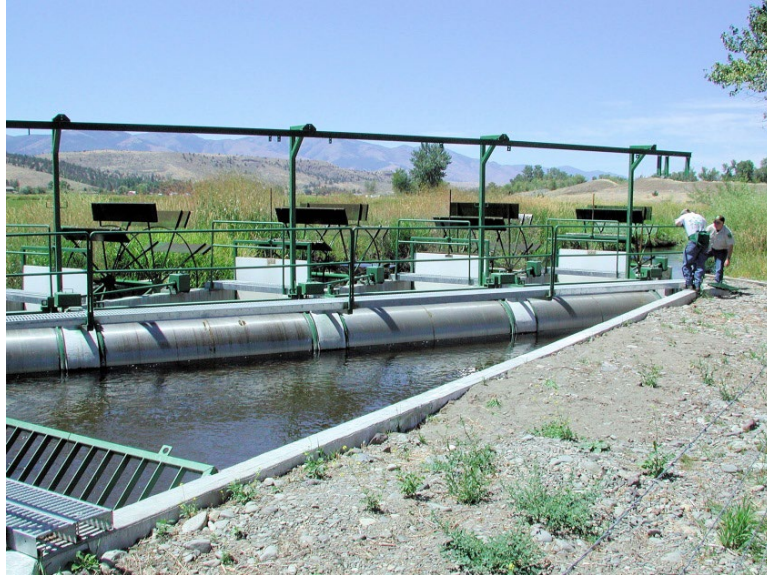
Figure 8-9 Rotary drum screens installed in a water diversion canal and operated (i.e., powered) by paddle wheels
