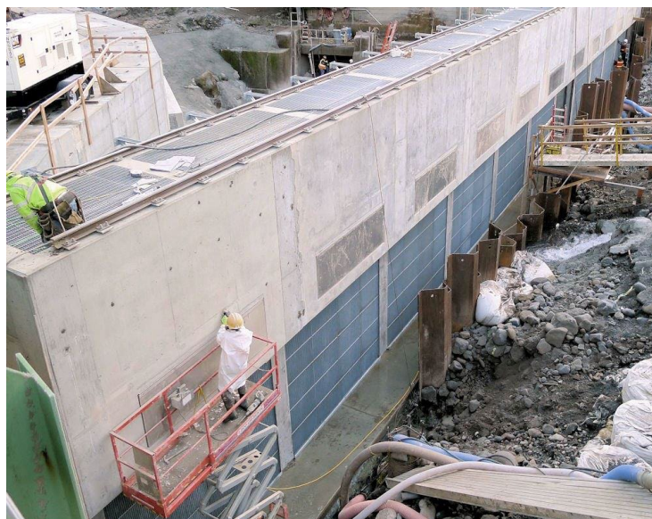
Figure 6-3. Picket barrier panels under construction at the Slide Creek tailrace barrier located on the North Umpqua River, Oregon
