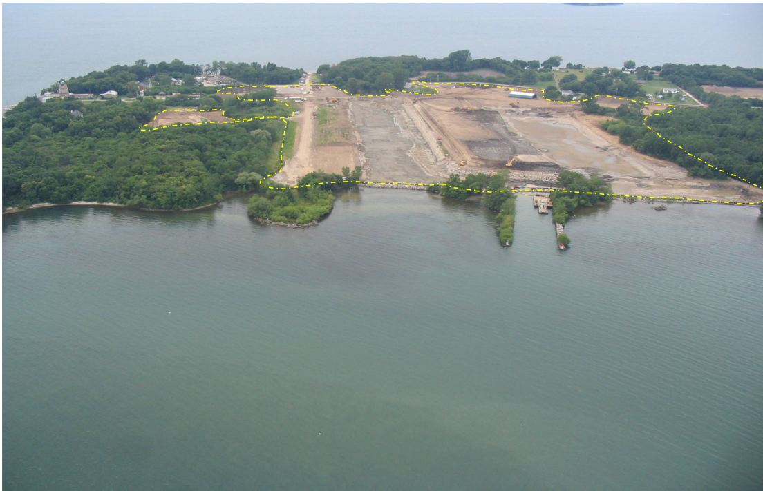
Figure 8. Aerial view of the Middle Bass State Park Marina Basin area during construction in 2008. The dotted yellow line highlights the area that was enclosed with a 3' tall snake barrier fence to exclude all snakes from the construction zone.
