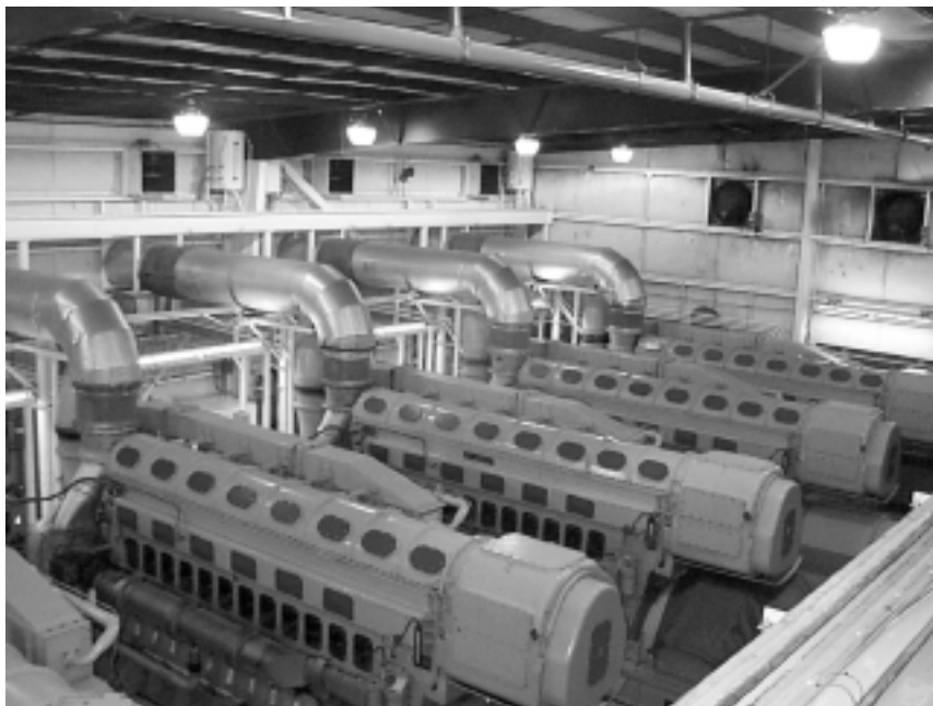
Figure 1. UniSea Powerhouse, Fairbanks Morse engine-generators nos. 4 through 1 (l-r).
