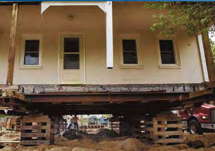
Norfolk, VA, East Ocean View home before being moved onto its new foundation, which will raise the first floor about two feet above the flood plain. Photo by the Virginian-Pilot
