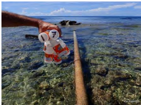
Fig. 4.2.30 Bairiki reef flat at point 17, exposed outfall pipe, looking South
