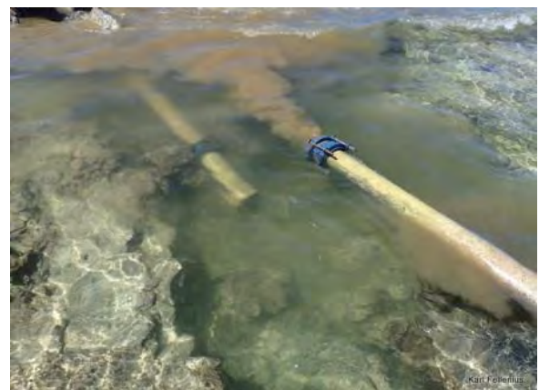
Fig. 4.2.33 Bairiki reef flat at point 25, end of existing pipe
