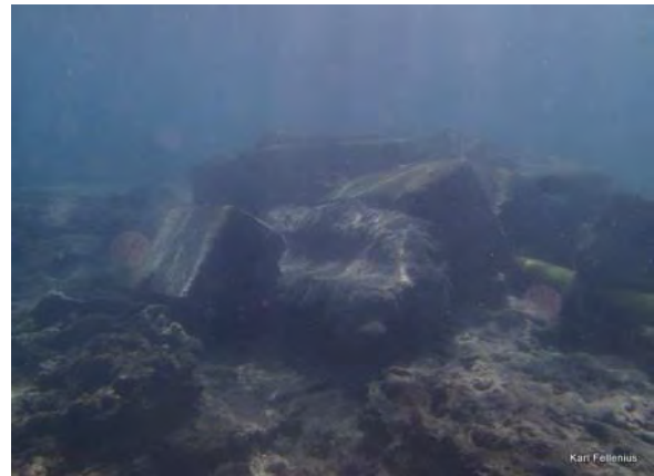
Fig. 4.2.45 From Bairiki end of existing pipe, looking Southwest to point 18, corrected height +0.6m
