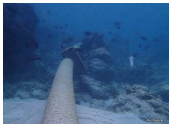
Fig. 4.3.45 From Bikenibeu 26m South of end of existing pipe, looking South, route along ↑ corrected depth 1.9m
