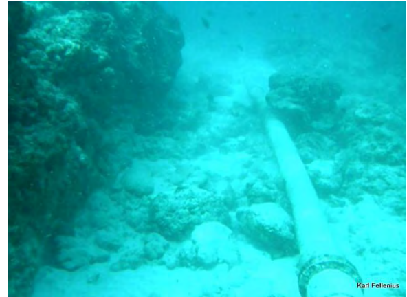
Fig. 4.3.41 From Bikenibeu 22m to 18m South of end of existing pipe, looking North, corrected depth 1.0m
