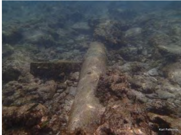
Fig. 4.3.36 From Bikenibeu 5m North of end of existing pipe, looking South, corrected height +0.4m
