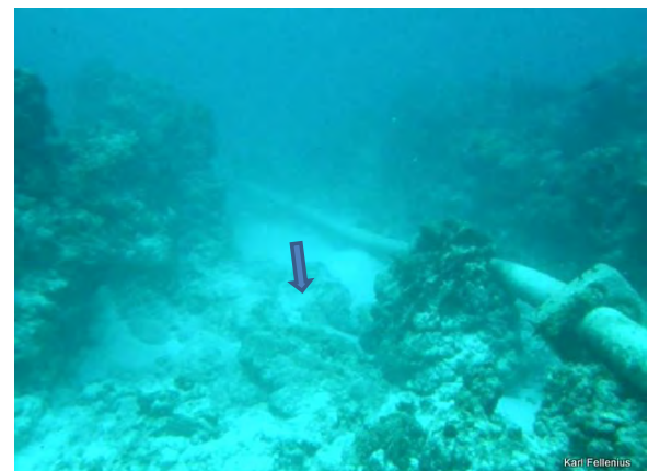
Fig. 4.3.43 From Bikenibeu 28m South of end of existing pipe, looking North, route along ↓ corrected depth 1.9m
