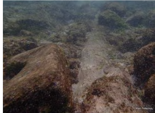
Fig. 4.3.37 From Bikenibeu 9m North of end of existing pipe, looking South, corrected height +0.4m
