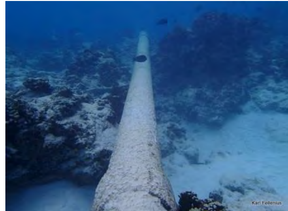
Fig. 4.3.47 From Bikenibeu 25m North of point 14, looking South, route along broken pipe, corrected depth 1.3m
