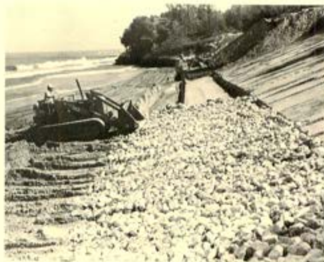
Equipment placement of large rock. It will later be covered with asphalt mastic.
