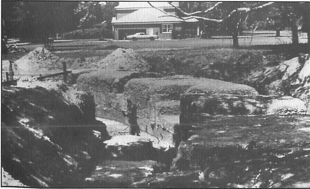
When a U.S.C.-Beaufort professor sought examples of tabby in Beaufort County, he found that it ranged from standing, occupied buildings to others which demanded excavation, as illustrated above.
