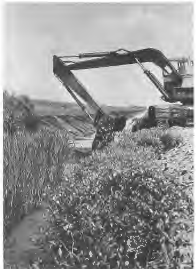
One of the farm's dozens of pieces of heavy equipment, this back hoe clears vegetation from a drainage ditch. The ditches will surround each square mile of the farm.
