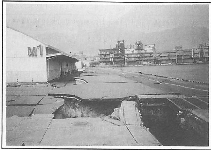
a) Looking North along East Face of Pier 1, at Location of Soil Settlement Adjacent to Steel Cell Caissons
