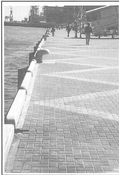
b) Wharf Surface after Earthquake
