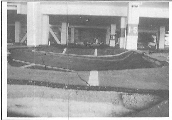
c) Fill Settlement
