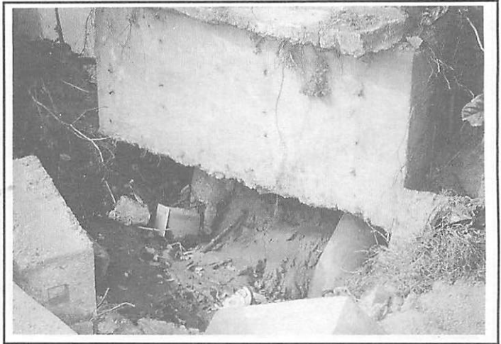
b) Damage to Lightly Reinforced Concrete Cylinder Piles Beneath Building in Foreground of a).
