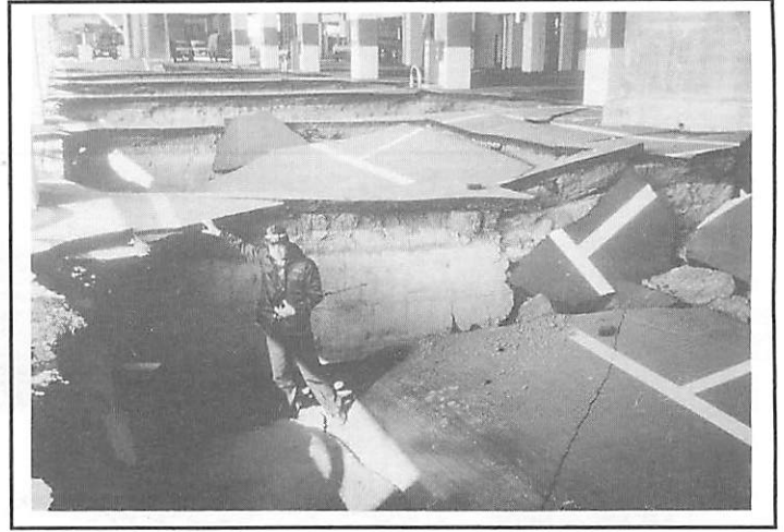
b) Fill Settlement
