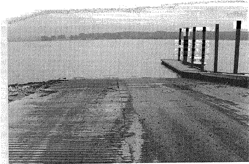
Figure 22 (a): The Weyerhaeuser courtesy dock is short, but in good condition. There are no cleats or tie-up devices on the ramp side of the dock.
