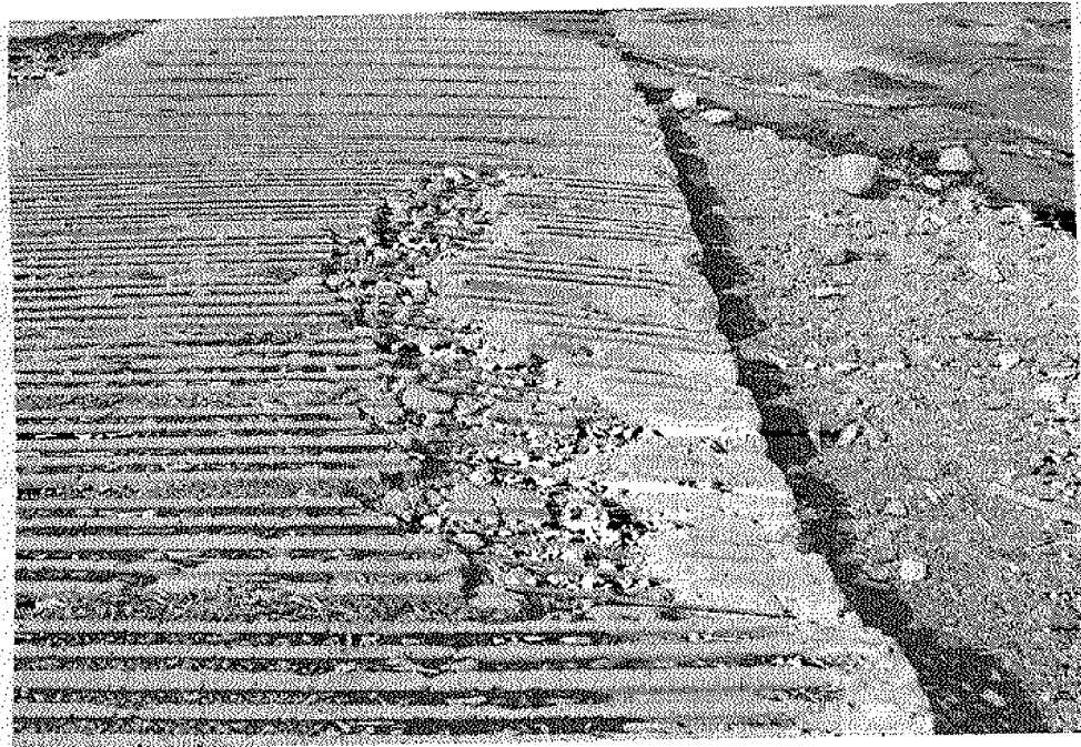
Figure 59 (b): A close-up view of the concrete plank launch ramp at Drano Lake. The ramp is structurally damaged.
