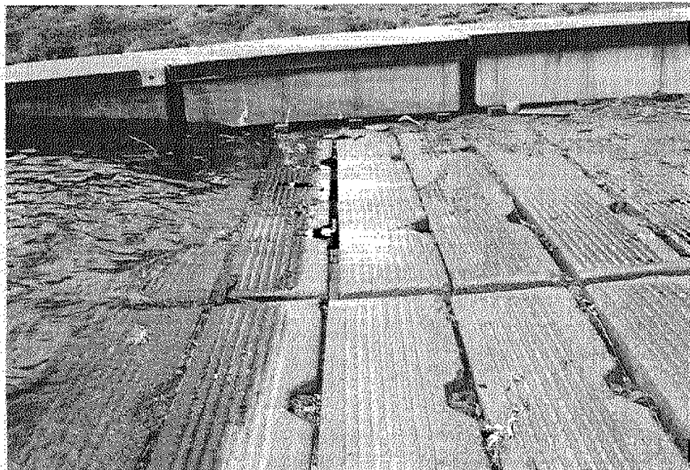
Figure 58 (b): Close-up view of the ramp. Some scuffing between the planks has occurred and should be repaired.
