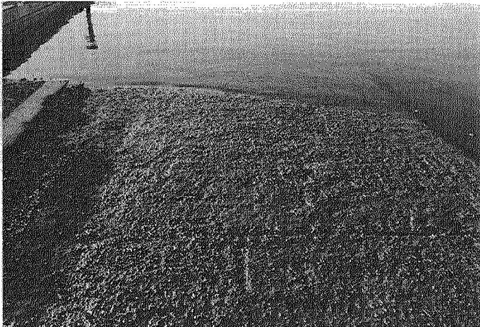
Figure 1 (b): Foot of boat ramp. Cracks and extensive pitting are apparent on the launch lanes.
