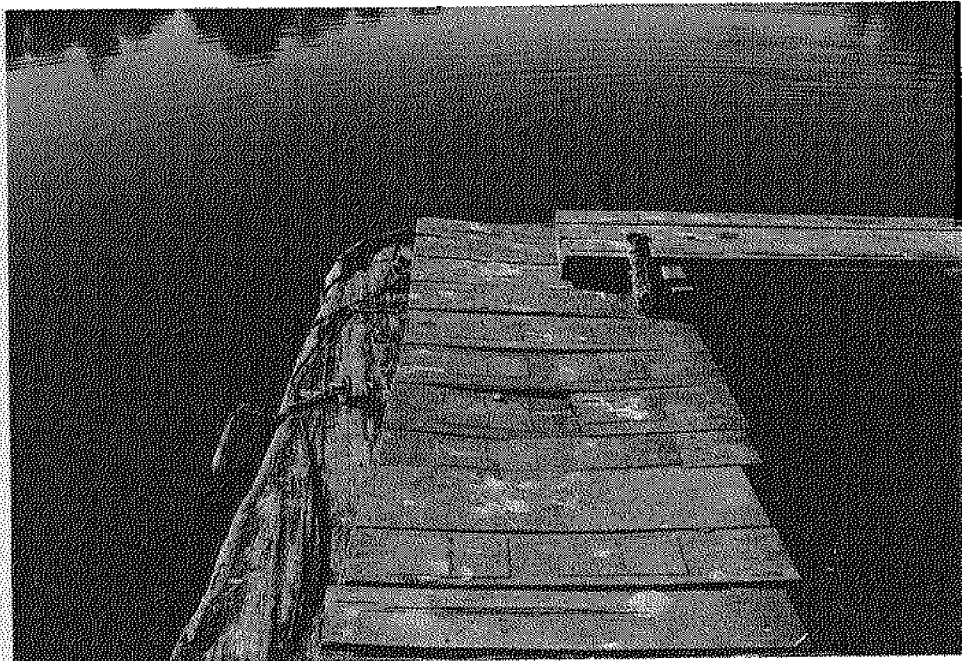
Figure 5 (b): Close-up of the courtesy dock. The boards on this log float are weak, patched, or broken.
