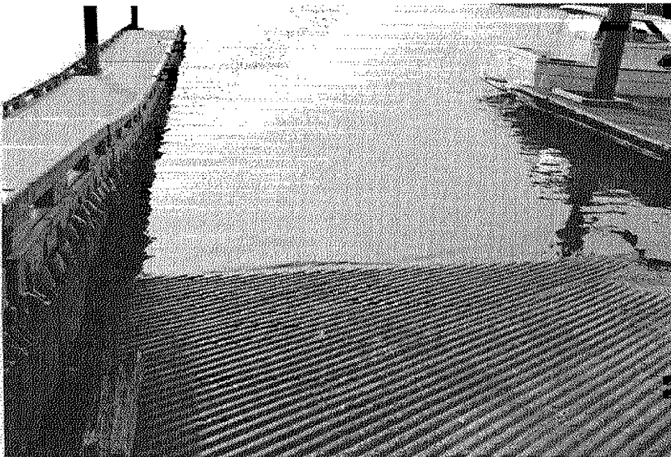
Figure 35 (b): A close-up of the ramp and courtesy dock. Both are in good condition. The dock on the right needs repair.
