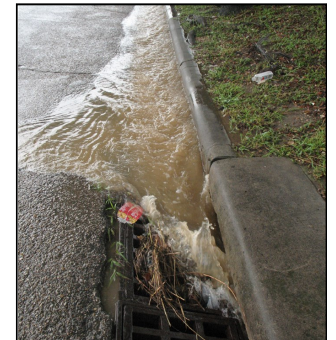
Stormwater running off an impervious surface. This water could be directed into a rain garden.
