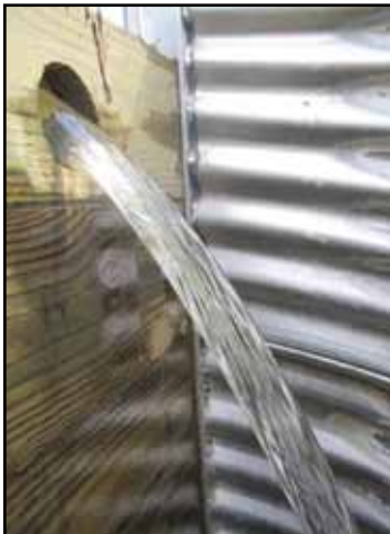
Flashboard riser, acting as a weir, with an orifice for slowly draining the temporary inundation zone. Photo Bill Hunt.
