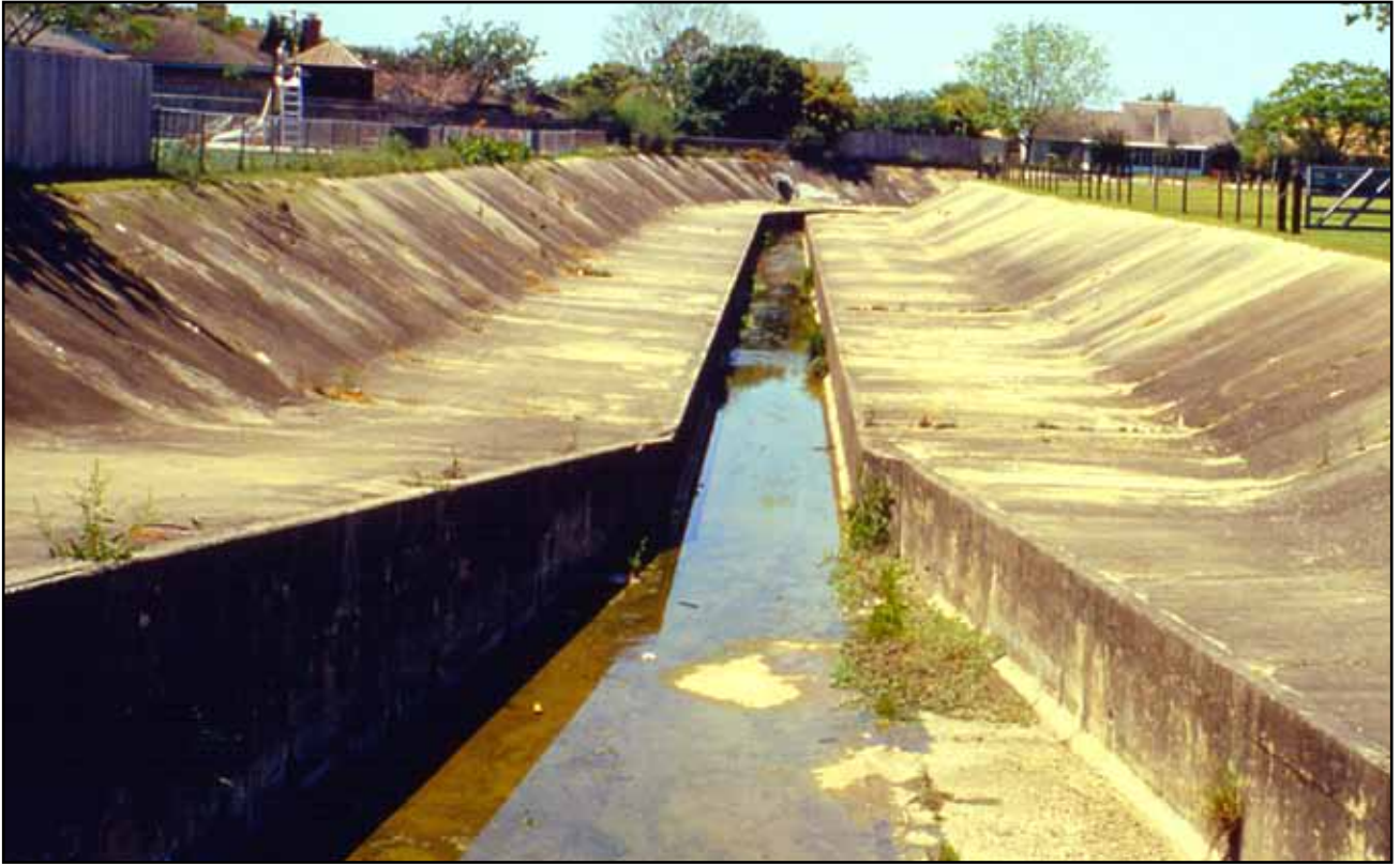
A single-purpose stormwater conveyance system. Note that this feature is along the backyards of these residences. A drain like this provides no water quality treatment and likely detracts from adjacent property values. Deer Park, Texas. Photo by John Jacob.
