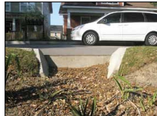
Debris removal from curb-cut needed
