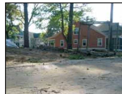
The construction site needs to be stabilized and the pervious pavers swept and vacuumed
