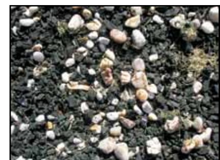
Loose aggregate that needs a top-coat applied
