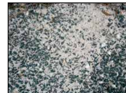
Sediment-laden Flexi-pave® indicating a need to jet-spray
