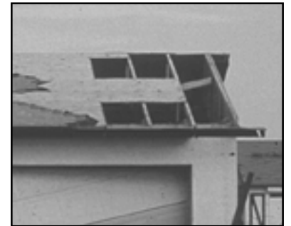
Typical roof sheathing loss.
