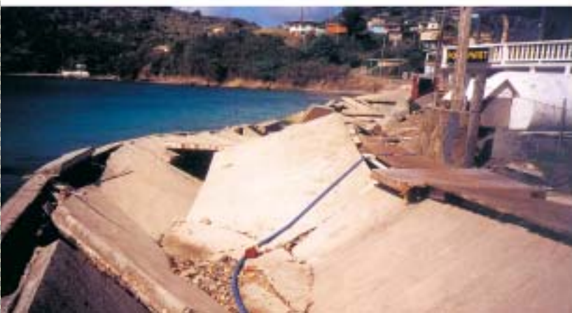
Hurricane Lenny caused serious damage to the coastal road at Hamilton, Bequia in 1999
