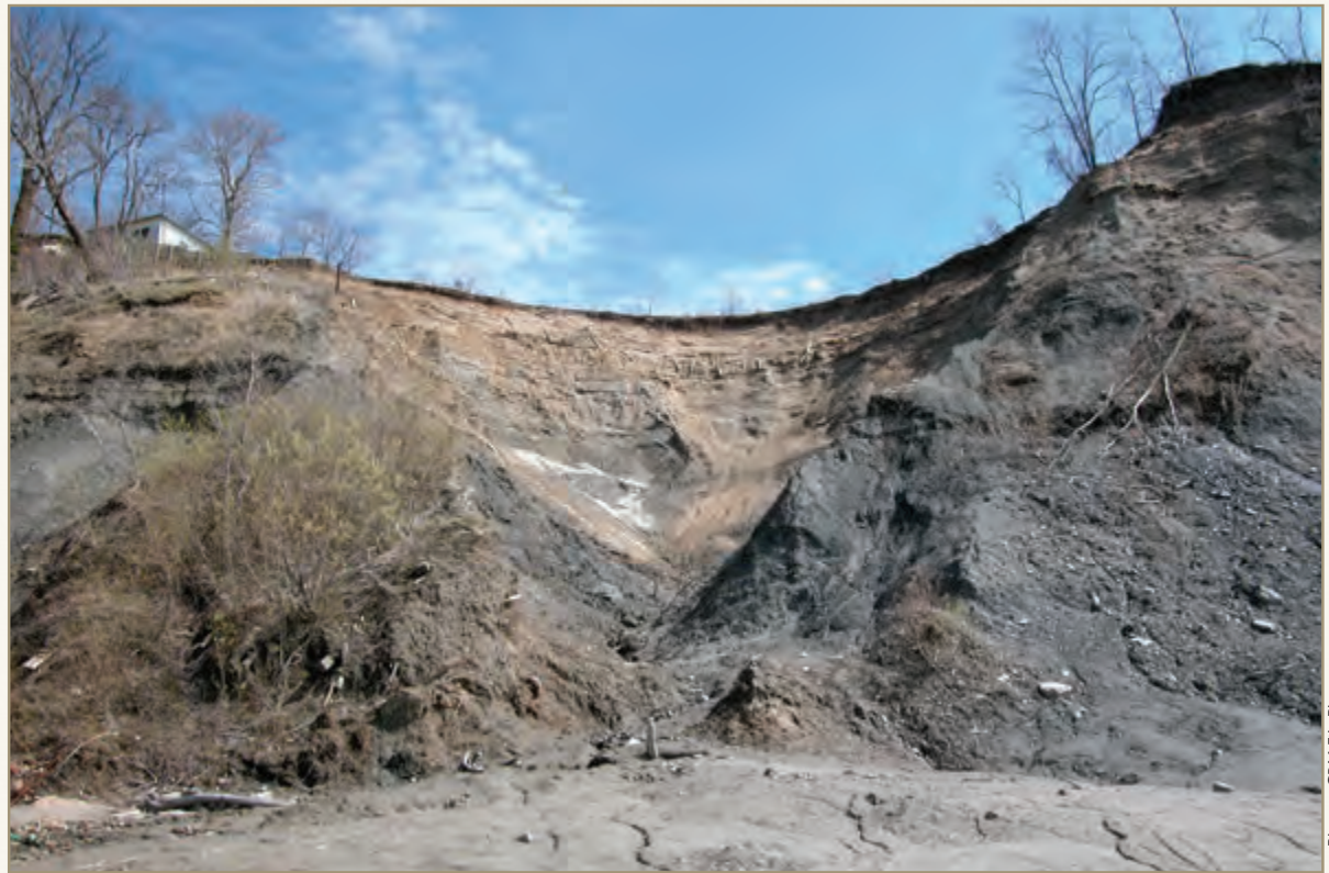
In this area in North East Township the sandy layer is especially deep, making it more susceptible to collapse.
