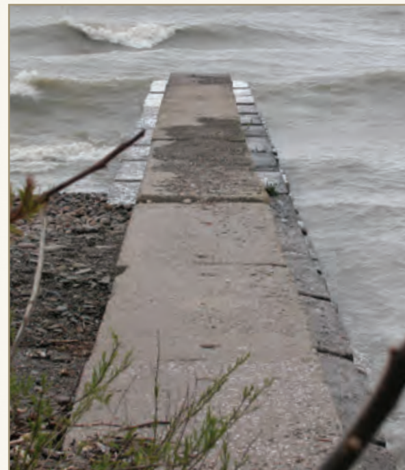
Sand and stones can be seen building up on the west (left) side of this groin.
