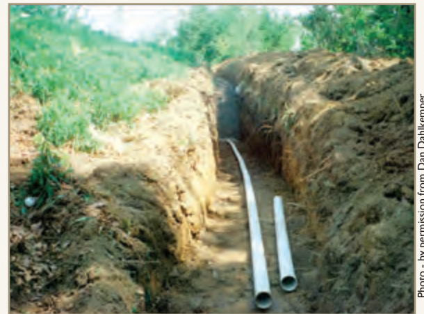
This is part of a drainage system designed to intercept surface runoff and groundwater. A drain (not shown) was installed in the low part of the yard.
