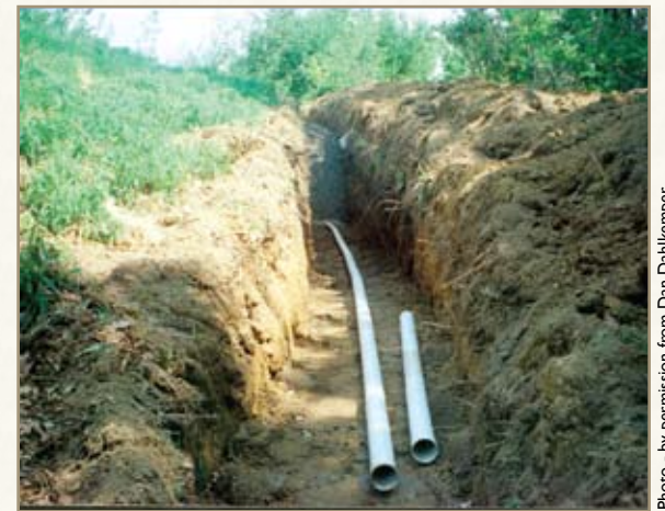
This is part of a drainage system designed to intercept surface runoff and groundwater. A drain (not shown) was installed in the low part of the yard.
