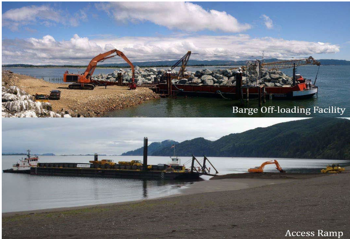
Figure 6. Example photos of island access for materials and equipment (Sand Island Pile Dike Repair Biological Assessment, USACE, 2020)
