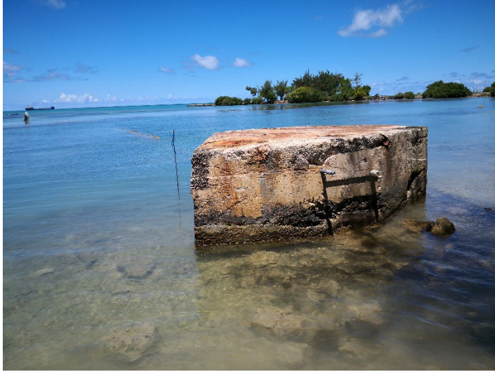
Figure E-3. Small cement platform near the coast considered to be part of the former Ship Ashore Restaurant that would be demolished. Credit: NMFS, 2021.
