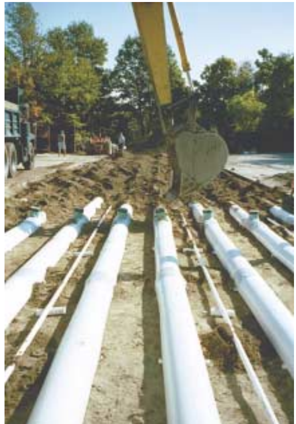
The shallow, narrow drainfield at the Purple Cat is installed into an island in the parking lot.
