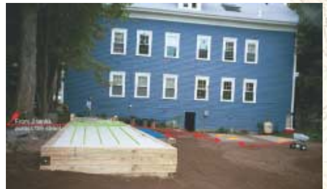
Completed system at rear of apartment building
