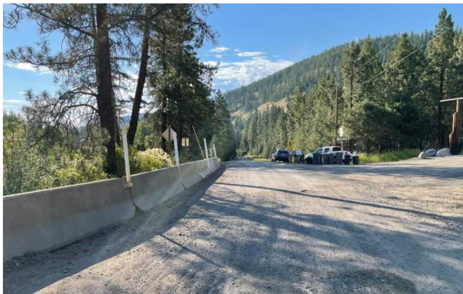
Photograph 3. Manastash Road at the erosion area looking southeast at single lane and current turnaround (July 1, 2021).
