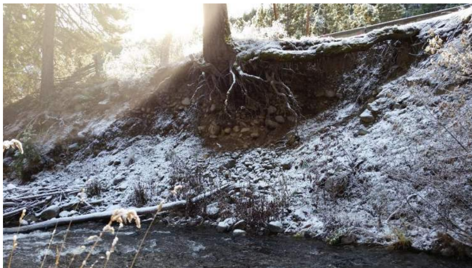
Photograph 1. Manastash Road erosion area, looking south towards the road (December 2016).
