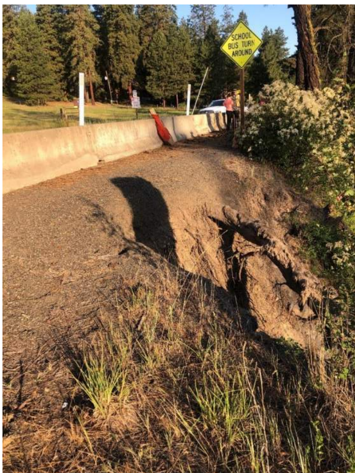
Photograph 4. Erosion area looking northwest (upstream) (July 1, 2021).
