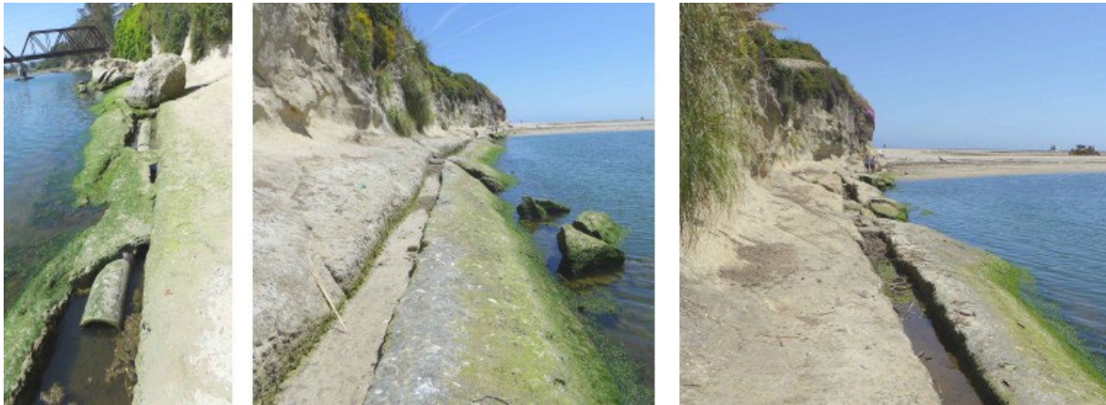
Figure 4. Portions of the existing trench and remnant pieces of the historic pipe within the trench along San Lorenzo Point.
