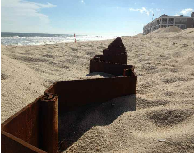
Figure 14. Sheet pile dune core (picture taken shortly after installation, before it is capped and buried by the dune), in Brick Township, New Jersey.
