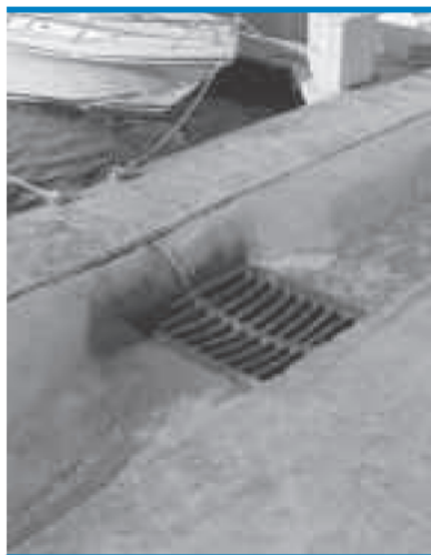
Stormwater inlet draining directly to marina basin.
