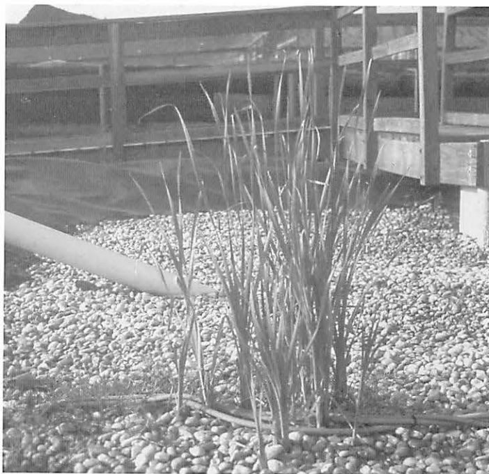
A constructed wetland in New Hanover County is a key part of its wastewater treatment facility.
