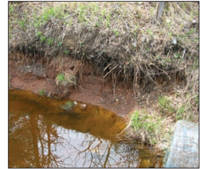
Figure 26: Side slope erosion (sloughing)
