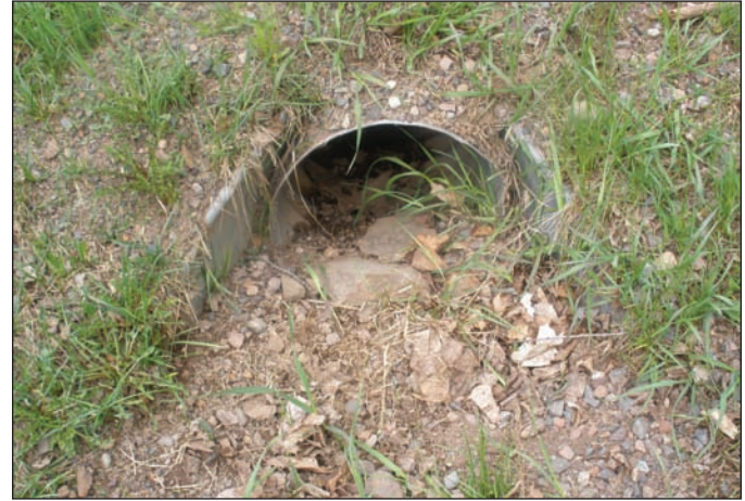
Figure 4: Debris blocking culvert
