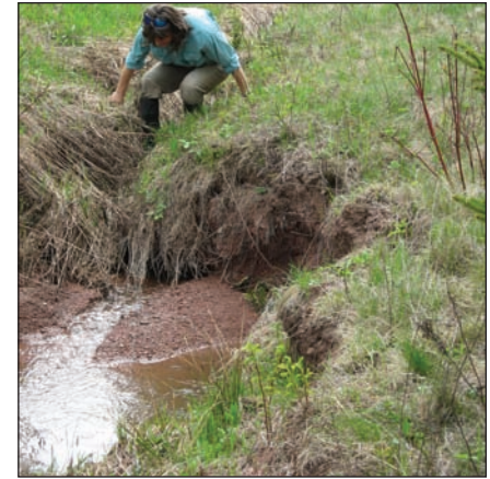
Figure 30: Headcut migrating upstream
