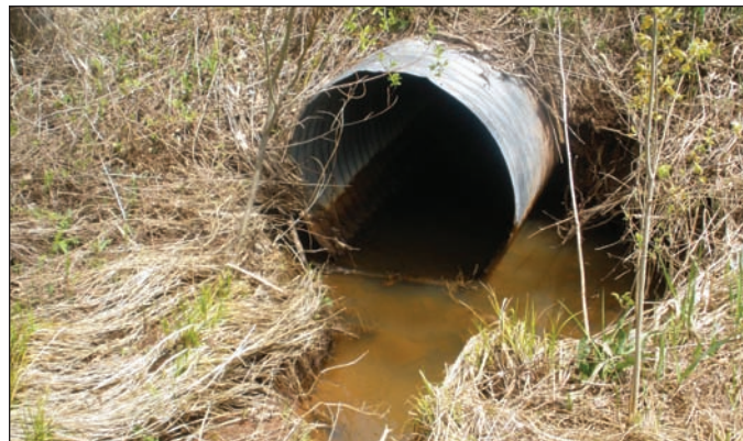
Figure 6: Minor erosion around culvert
