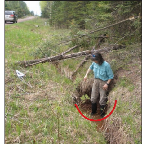
Figure 36: Example of a ditch you don't want to dig- a U-shaped ditch with vertical sides
