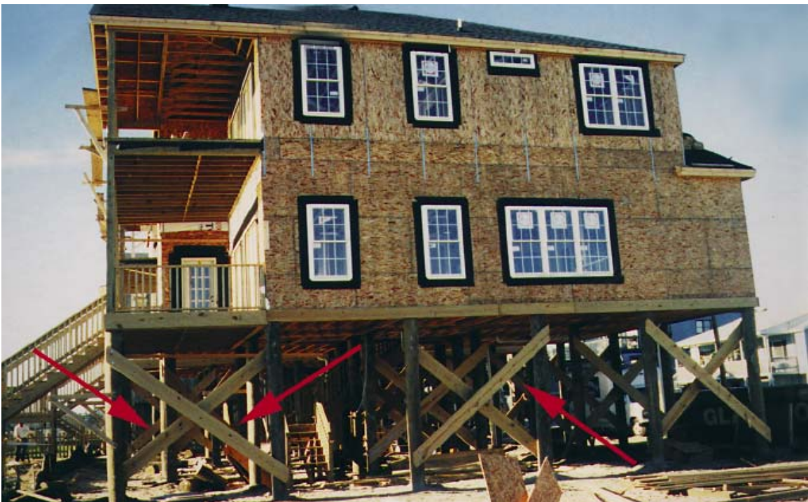
Figure 4-11 - Cross Bracing. From FEMA CCM, 2000. Cross bracing can also add strength and rigidity to piers or columns, but mixed results in actual field conditions may warrant increasing strength by other means (e.g., stronger column material or greater widths).
