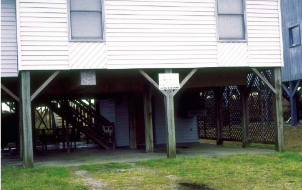
Figure 4-12 - Knee Braces.- Another way to increase strength and rigidity of piers and columns is to utilize knee bracing. Because there are no obstructions at grade, scour risk is reduced. Since bracing is near the top only, the potential for catching debris is reduced. However, knee braces are not as strong as diagonal braces and shear at the top is increased. Also, it may be difficult to brace only in the direction of flow. From FEMA CCM, 2000.
