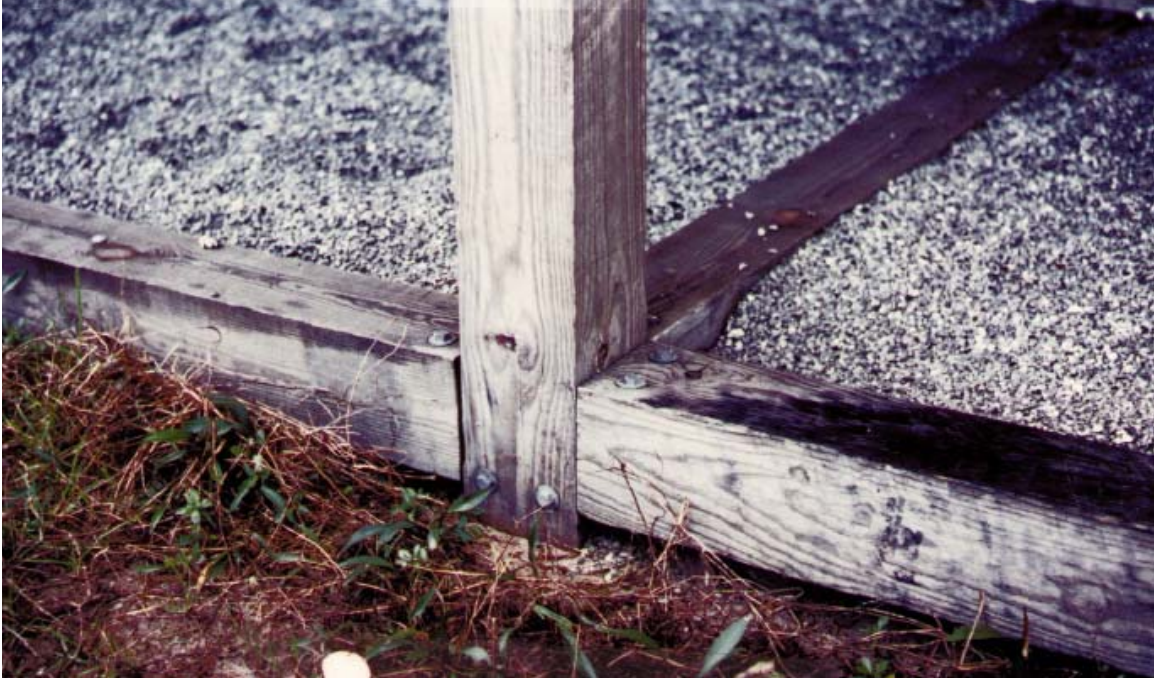
Figure 4-10 - Grade Beams. Grade beams can be used to tie the structure at the foundation and are especially useful if there is localized scour or erosion. In this case the grade beam may prevent localized collapse. From FEMA CCM, 2000.
