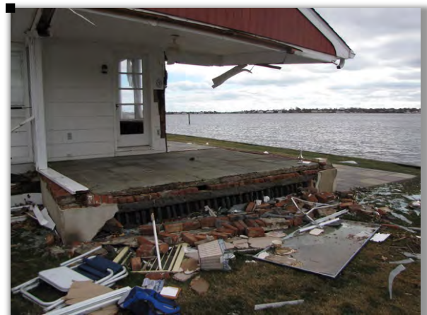
Figure 3.7.1:1 Sandy's wrath on Little Silver Point Road in Little Silver, NJ
