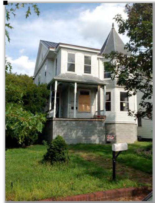
Figure 3.10.3:5 - An elevated home in Portsmouth
