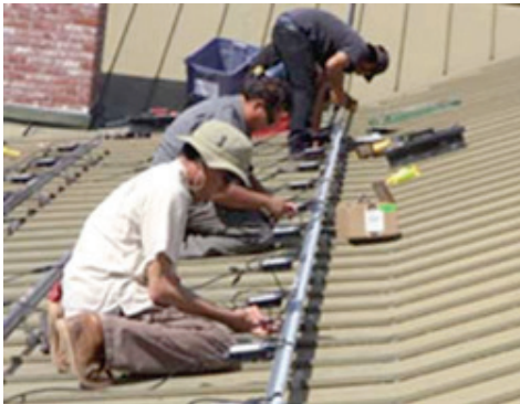
Residential Solar Installation. Source: SYCEO
