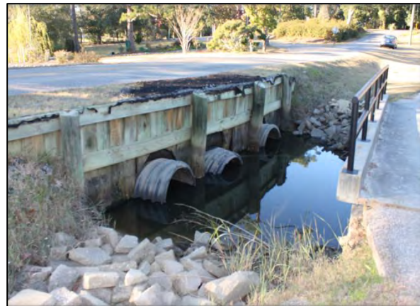
Figure 1. Poorly functioning culverts such as this prevent adequate water exchange. Photo credit: Meg Goecker
