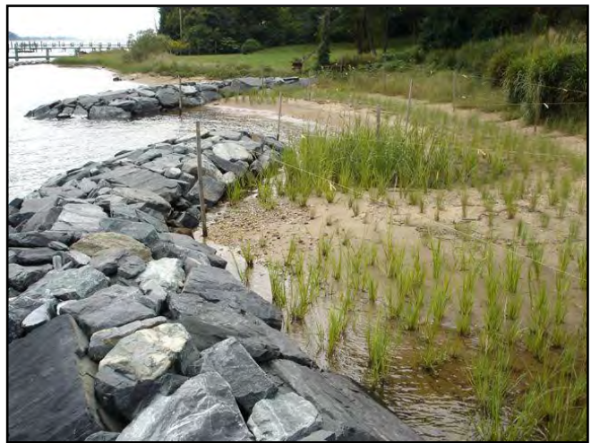
Figure 1. A representative example of a constructed living shoreline using rock, vegetation and clean sand fill.
