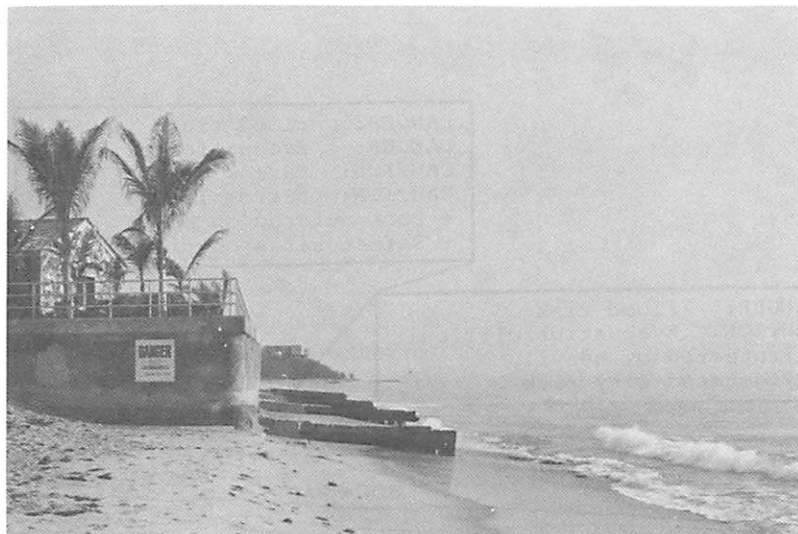
Fig. 4.45. Seawall and groin in front of a too-close-to-the-beach development. Juno Beach south of Jupiter Inlet. Photo by Bill Neal.
