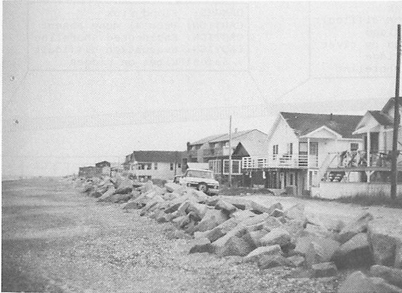
Fig. 4.10. Cottages on Fernandina Beach “protected” by a revetment. Photo by Barb Gruver.
