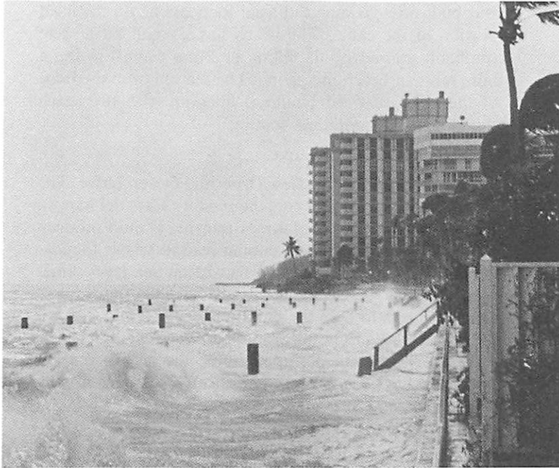
Fig. D-4. View along the seawall of the Key Biscayne Hotel during a winter storm in January, 1982. Note how the seawalls completely reflect incoming waves. This tends to move what sand is near the shore back seaward off the beach. Hence seawalls, while protecting basic structures built close to the beach, tend to destroy the beach. Of course the beach was the reason the buildings were built there to begin with.
