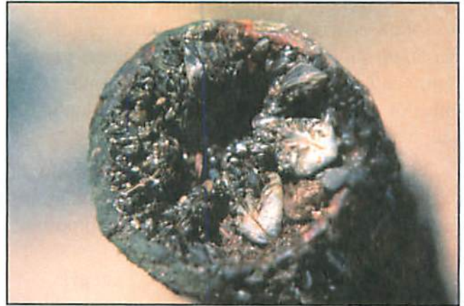
Figure 5. Water intake pipe clogged with adult zebra mussels.
