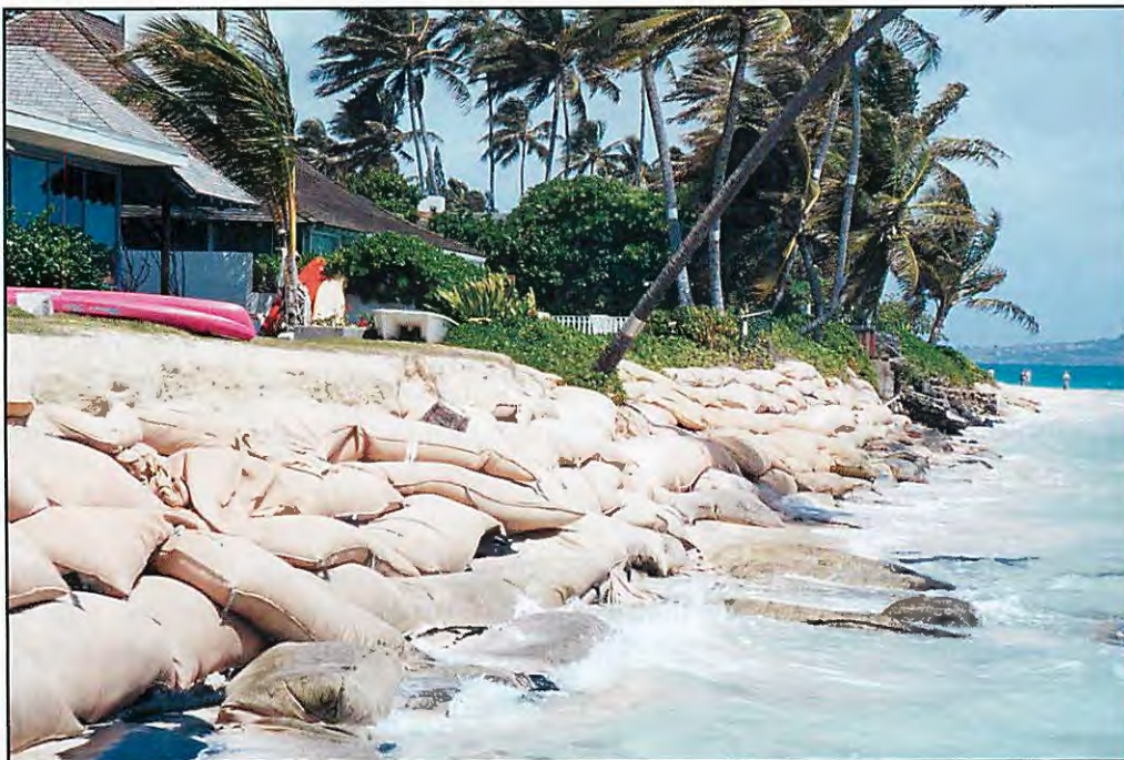
Figure 12-3 – Large Sand Bags for Erosion Control, Oahu - Large bags or geotextile tubes are filled with sand, placed parallel to the shoreline and stitched together to form a barrier against erosion. Damaged and displaced sand bags are in the water.
