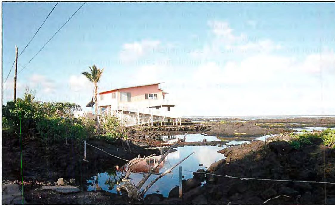
Figure 3-12 – Kapoho Vacationland Subdivision, Hawaii - Subsidence of land at the Kapoho Vacationland Subdivision has resulted in homes being exposed to flood waters and wave action during monthly high water levels. Homes have been elevated to mitigate flood damage.
