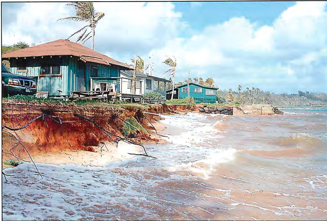
Figure 9-6 – Aliomanu Bay, Kauai – Erosion of the shoreline and the soil profile threatens the house and impacts water quality. These impacts can be mitigated with the proper setbacks and by using sand that meets the standards in Figure 9-5, instead of soil as fill in the erosion zone. Photo by Dennis Fujimoto of Garden Island News
