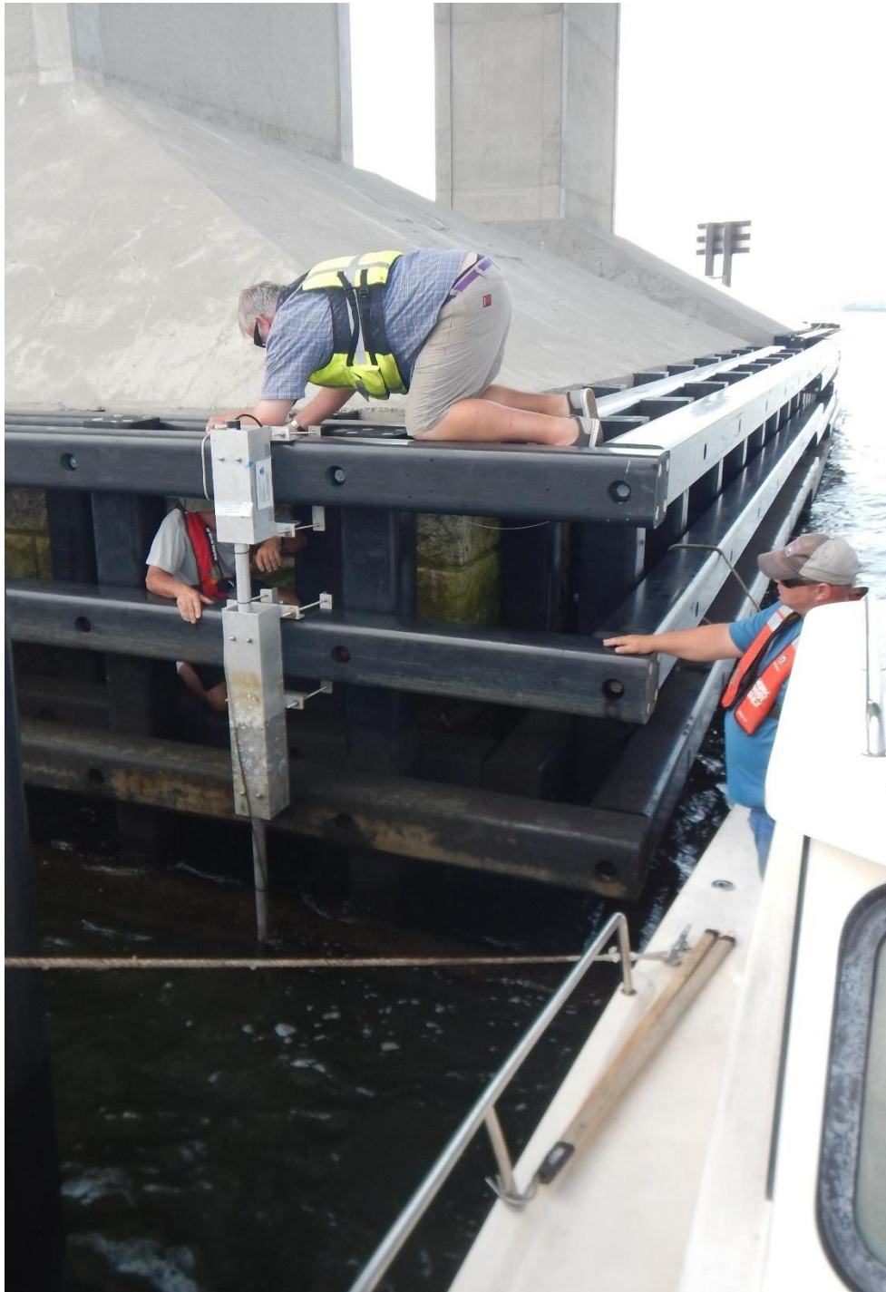
Figure 3-4. Horizontal crib mount being installed. ADCP is held at the bottom of the pole, below the surface.
