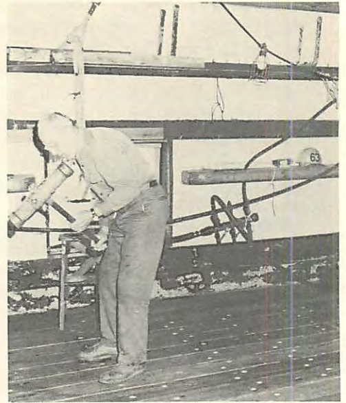
Caulking the new spar deck forward. Planking is fir 4½ inches thick. A temporary roof has been installed over the work area.
