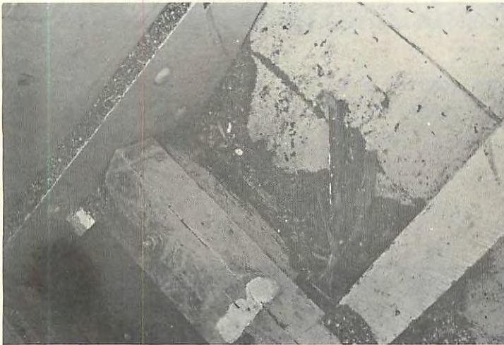
Accumulated dirt and moisture trapped beneath the leaks across her stern rotted out the lower framing of the transom.
