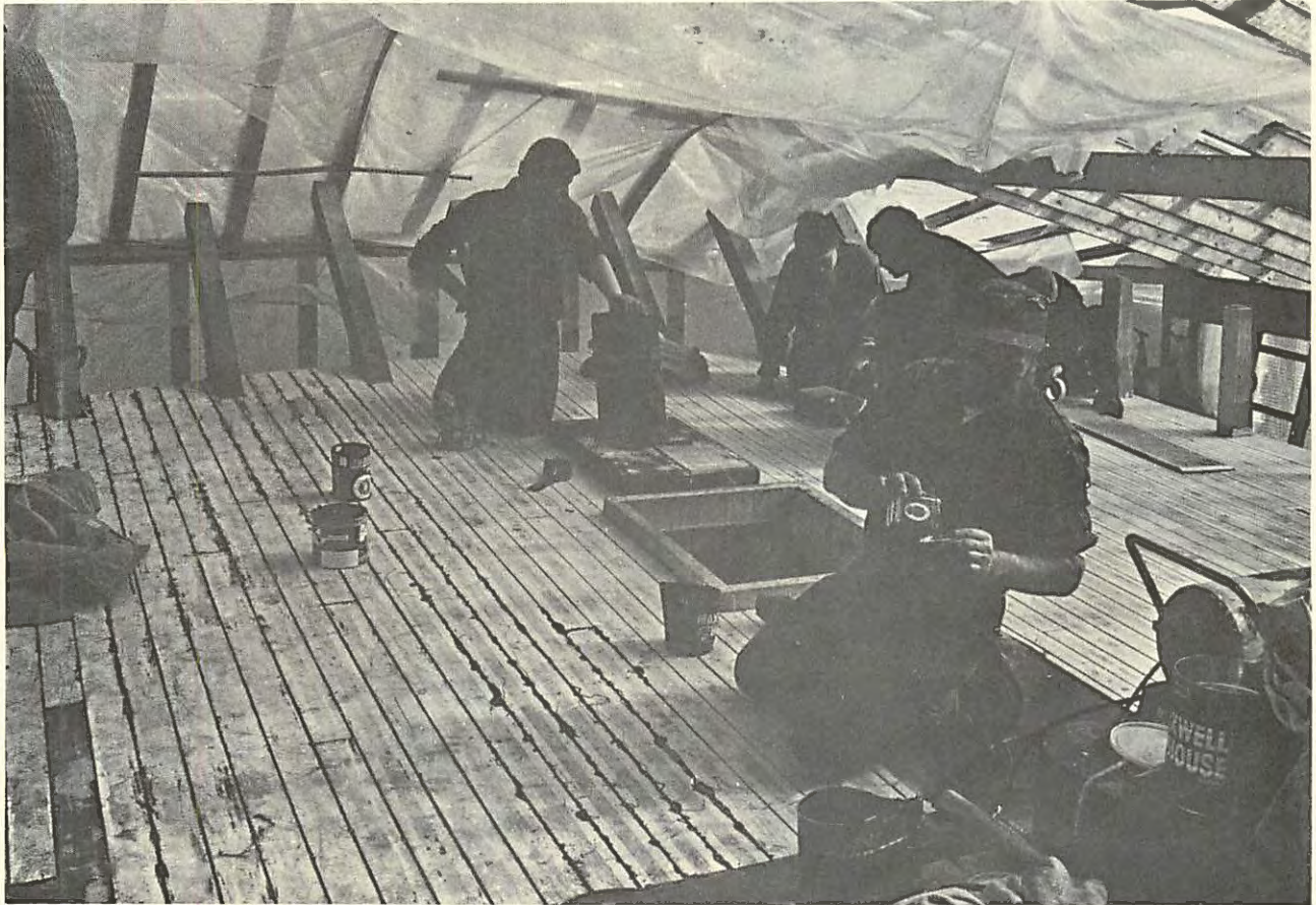
The new decking was run all the way aft, eliminating the covering board which originally ran across the stern. This arrangement should be easier to keep watertight.
